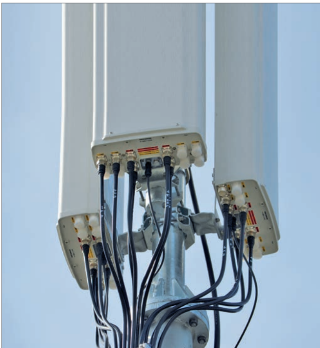
Installation of 3 x 12-port Kathrein FlexRET antenna 80010899 with 6-way Site Sharing Adapter
