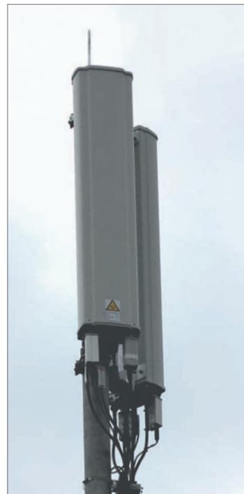
Antenna site for LTE 800 and UMTS 2100 with two Kathrein 4-port antennas and RCUs for each system
